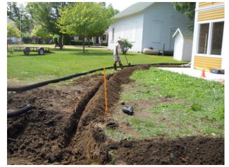
Drainage System –Al Horton, Bob Graham, Fred Farkas, Don Allen, and Dick Waters
